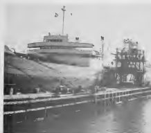
THE NORTH side of No. 1 Finger Pier underwent a major renovation recently. Timbers along the length of the pier were replaced and where mooring dolphins were located, new sleeves for
